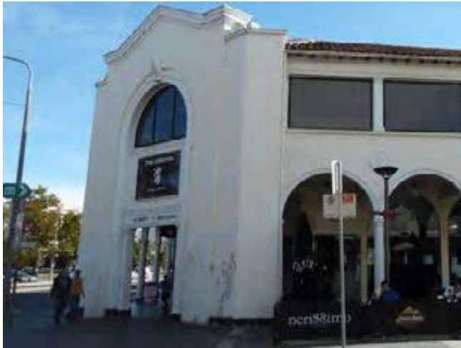
Figure 46. Paint and render problems on the Sydney Building Source: Duncan Marshall 2011
