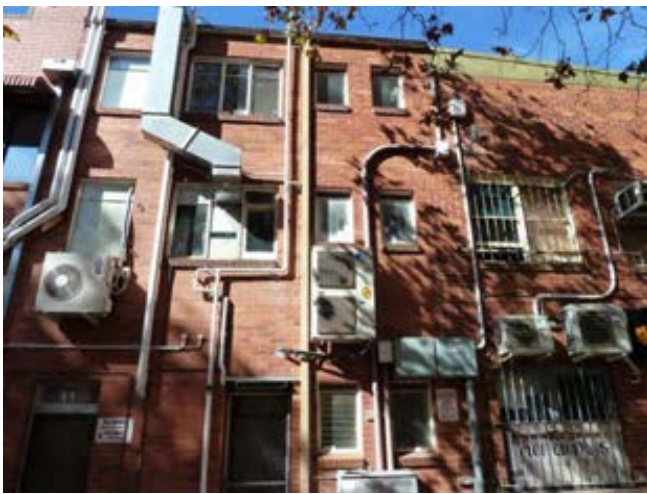
Figure 19. Sydney Building courtyard – note wall mounted services Source: Duncan Marshall 2011
