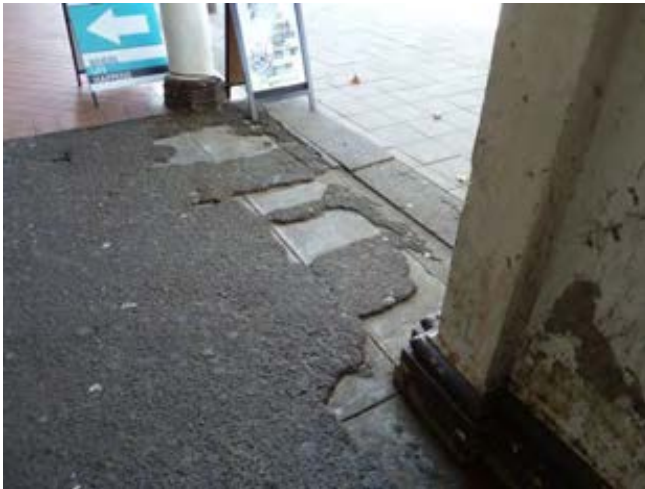
Figure 7. Section of bitumen paving in colonnade of East Row – note original concrete finish underneath
